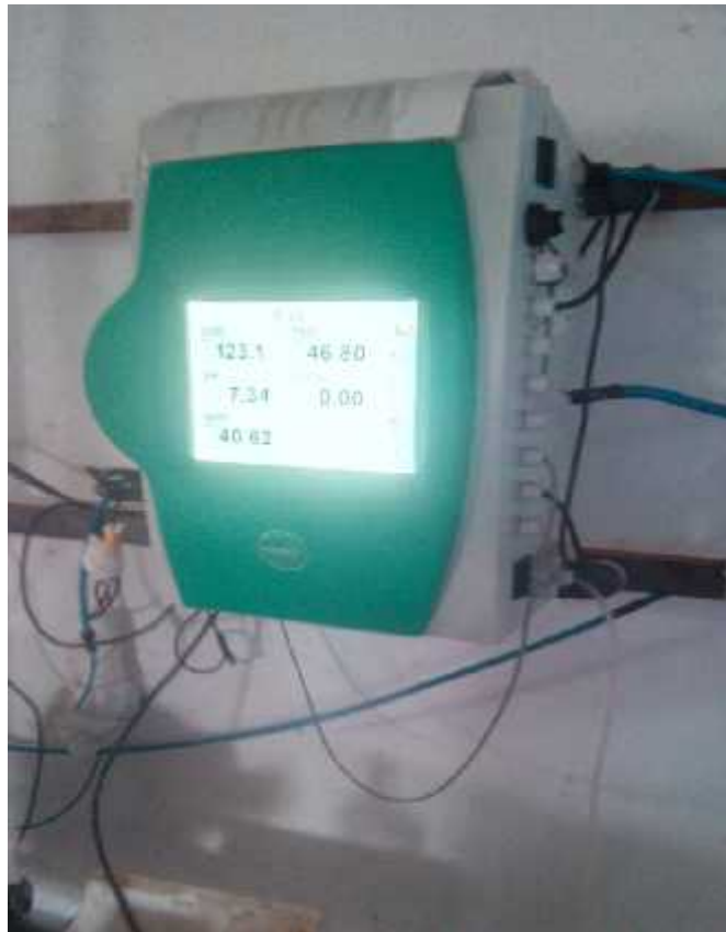
Photo.8 - ONLINE EFFLUENT MONITORING SYSTEM FOR ETP
