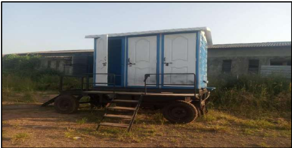
Photo.3 – Provided Sanitation Facility to the Contractor Labors
